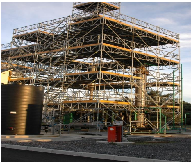
Figure 1 : The SOBEGI site in Lacq, France
